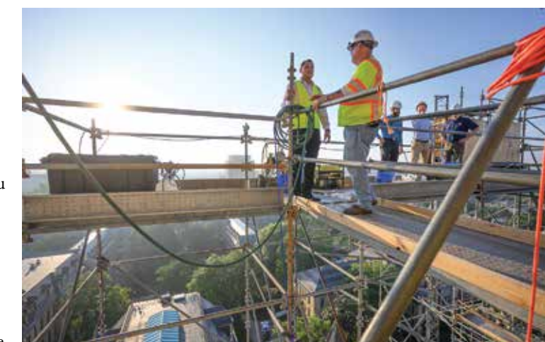
Tony Polotto walks high above the Main Building on the scaffolding surrounding the tower and Dome during the 2023 regilding project. (Photo by Matt Cashore/University of Notre Dame)
