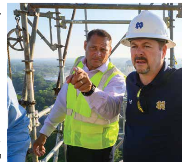
Tony Polotto talks with Mike Daly, senior director of project management, during a visit to the Main Building regilding and restoration project. (Photo by Matt Cashore/University of Notre Dame)
